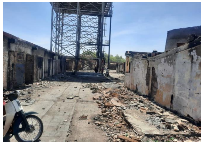
H: Overhead water system damaged by the fire incide
